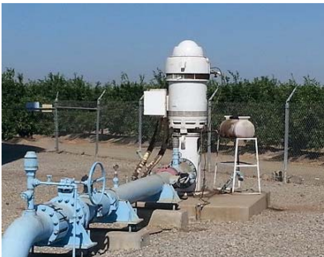
Figure 7. Typical District-Owned Groundwater Well
