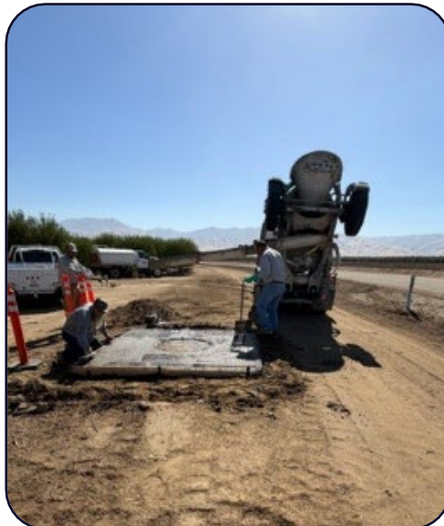
Cement Pads for Air Valves on B-2 & C-3 Laterals
