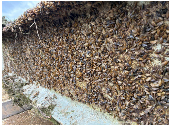
Traveling Water Screen, 850 Canal D-Reach
