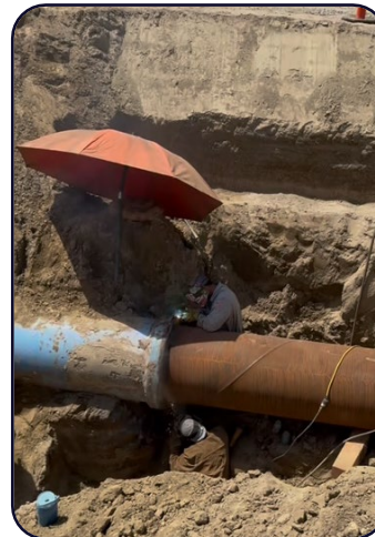
8P Lateral Leak
